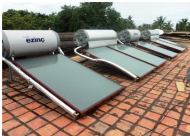
Solar panels at Travellers Beach Hotel
