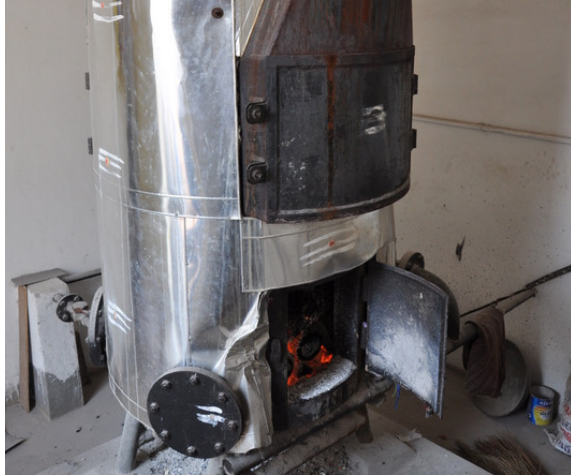
Centralised energy efficient boiler established at SJP saving 40% of energy consumption and Rs. 10,000 per month
