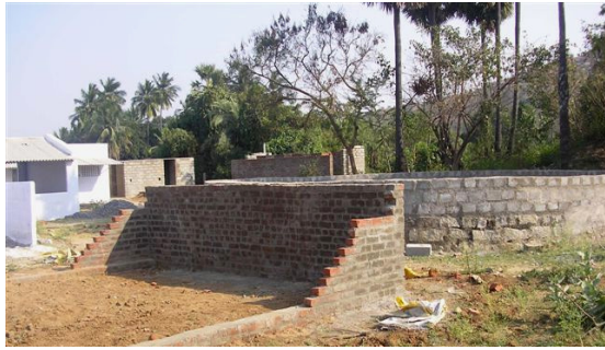
Construction of housing facilities at Foods and Inns. In the background on the left new dormitories can be seen, in the foreground a dormitory is under construction and in the background on the right, the well with its new elevated wall can be seen.
