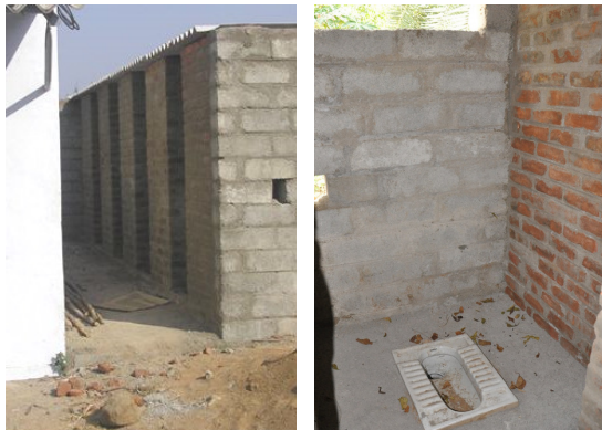
Toilets under construction at Foods and Inns. Before only four toilets existed and were to be shared between male and female workers. Now, sufficient toilets as well as showering facilities have been constructed for separate use between male and female workers
